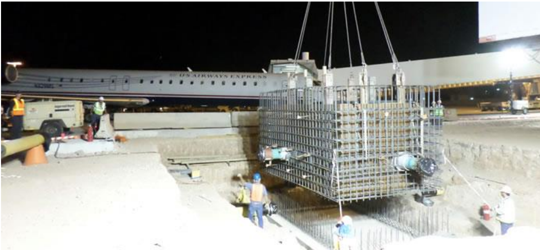
Inset 5.29: Example installation of a prefabricated fuel skid with valve chamber
